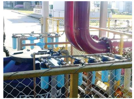
Figure 2: Pilot system, two treatment trains with 5 micron-filters installed
