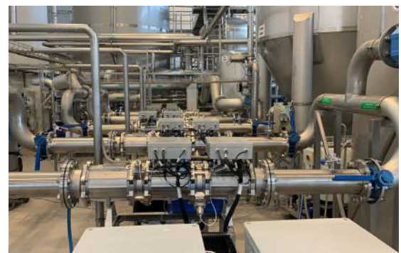
HOD™ UV provides product water disinfection and ozone destruction, reduces maintenance and operating costs at PepsiCo Domodedovo, Russia.
