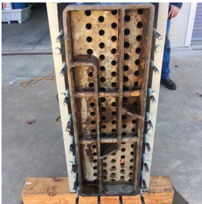
After photo of heat exchangers, with scaling noticeably reduced.
