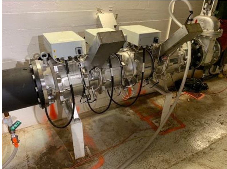
Atlantium's Hydro-Optic™ (HOD) UV demonstration unit installed at OPG DeCew II Generating Station.
