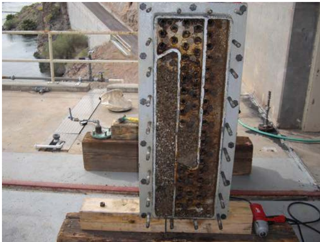
Before photo of Parker Dam heat exchangers, with significant scaling
