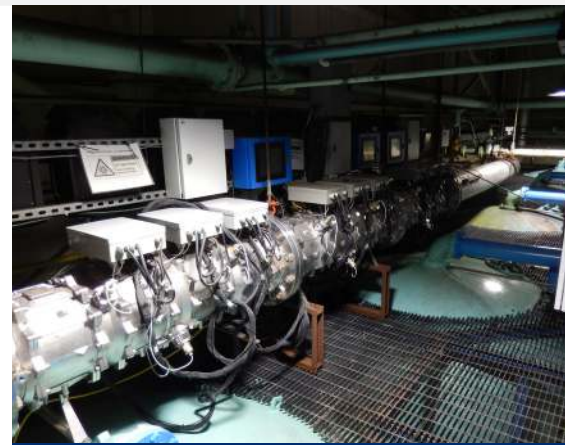
Hydro-Optic UV system on Georgia Power's Plant Bowen reverse osmosis unit
