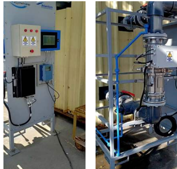
Figure 3: Installation skid HOD™ UV with RZ163-11 HP, 2.3 kW equipment
