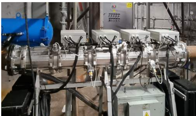
HOD UV system consisting of a filter plus the HOD UV system installed in the cooling system of generator unit 4 of Governador José Richa Power Plant
