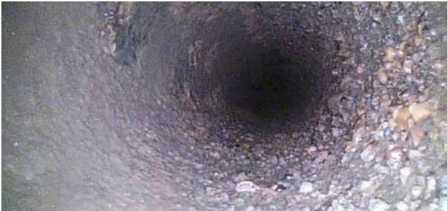
Boroscope photo without mussels, mud, or hydrozoa in the bearing pipe after the HOD UV system. The stains shown in the photo correspond to old corrosion in the piping.
