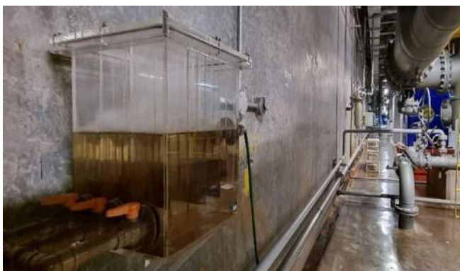
BioBox installed in the cooling system of the Governador José Richa Power Plant
