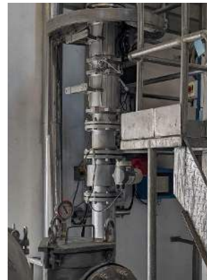
Atlantium RZ163-11 vertical system installation in 2014 with 250 gpm flow rate
