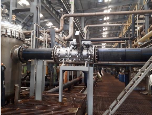
Figure 3. Seawater Desalination Facility With MP-UV Installed
